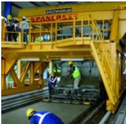
Fig 4: The Spancrete GT 240 slipformer is producing 150,000m 3 hollowcore slabs per year on two beds 115m long
