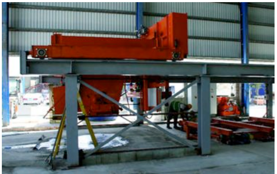
Fig. 8: The concrete distributor is served by a forklift currently. Later a flying bucket conveyor system will speed up the delivery of the concrete.
