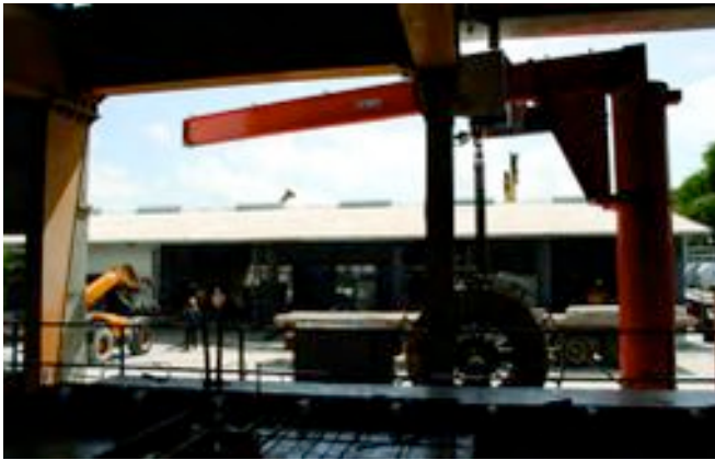
Fig. 14: KRB straightening and shear lines are used for the rebar processing. After preparing the reinforcement in the other hall, it is brought to the pallets by crane from outside
