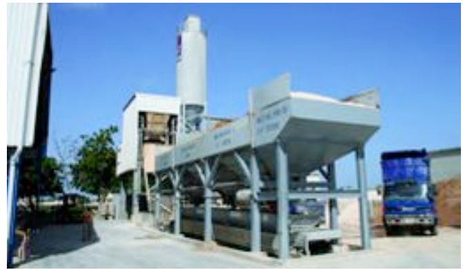
Fig. 15: The mixing plant from Elematic is serving both the dry cast and the wet cast operation
