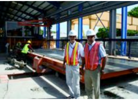
Fig. 10: The tilting station U1 is designed to enable other pallets to bypass this station during the demoulding process. Mark Maloney MD Preconco (left) and Mathias Reymann, President Ratec, are convinced that the circulation process for precast production is an optimal solution for a production of modern precast concrete walls.
